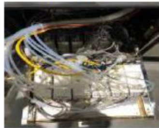
PR Pump Area (Front)
