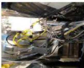
PR Pump Area (Rear)
