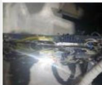
PR Pump Area
